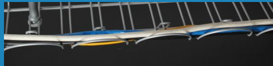
Cable tray with cables
