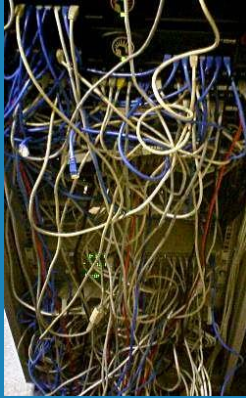
Poor cable management
